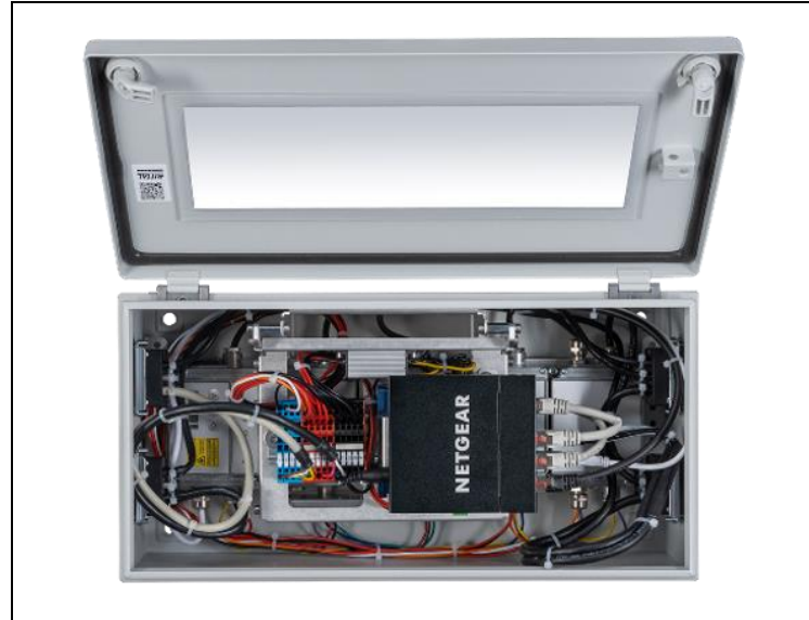
Figure 22: Control cabinet open
